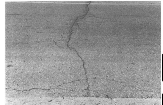
Moderate (Multiple) Transverse Crack
