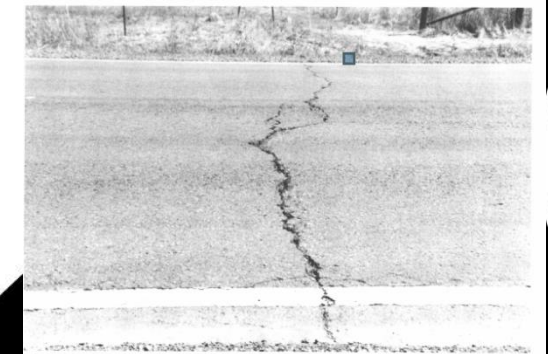
Severe Transverse Crack with Spalling
